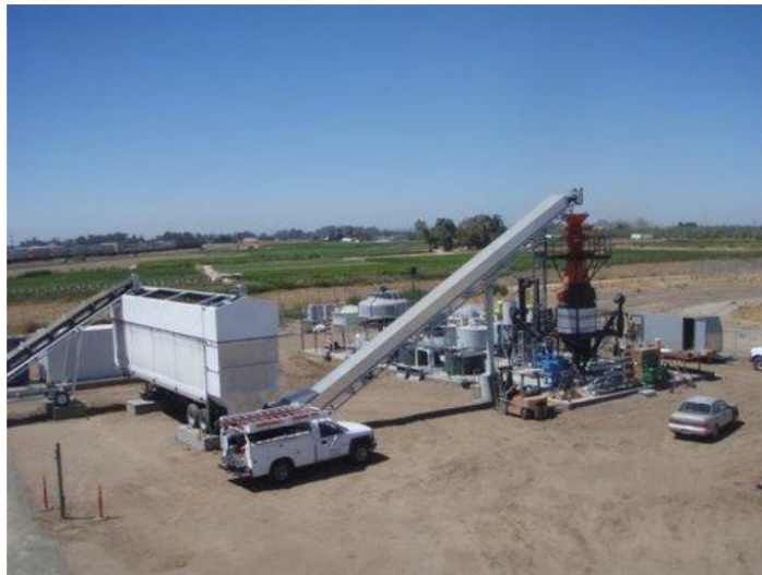
Figure 3 – A P500 installation in California
