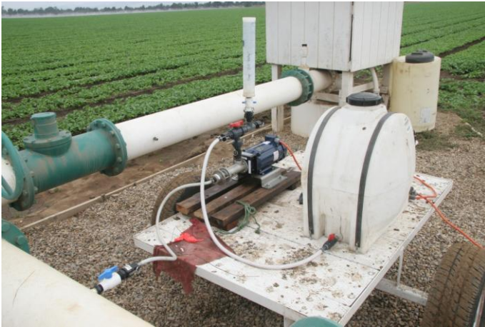
Figure 2. Trailer outfitted for injecting liquid PAM into the main line of an irrigation system using an auger metering pump.
