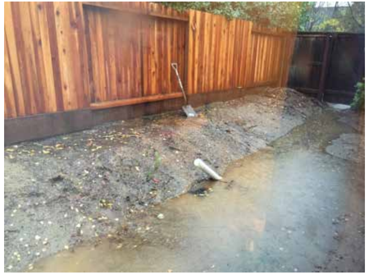
Before (above): High clay content soil was not planted or covered with mulch. During heavy rain, the water pooled around a drainage basin which took the storm water to the street.
